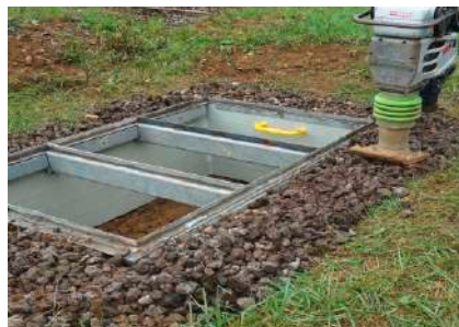
5. Fill the excavation flush up to the frame and compact with a vibratory tamper.
