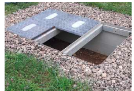
6. The GRP cover plates are installed with a cable junction box lifter.
